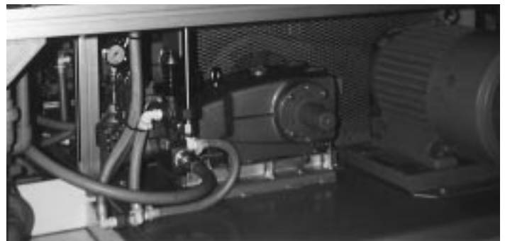
Closeup of Power Unit drive source.
